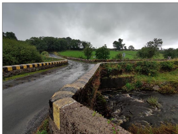
Figure 7 - Bridge C6 towards Dungarvan Substation
